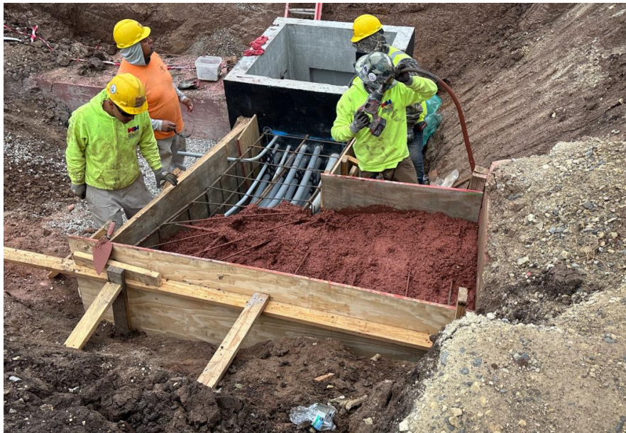
Concrete Encased Electrical Conduit
