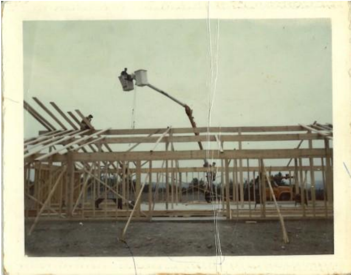
Figure 4. Photo of the PAL Building (then Ski Lodge) being built at Essex Woods. Date of photo is unknown, and the photographer is unknown but assumed to be Rolland Perry.
