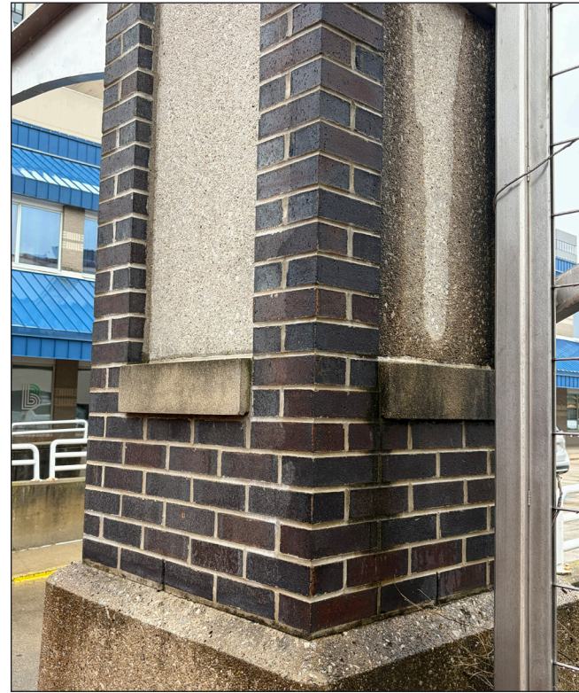
Brick and cast stone features can become stained over time. Cleaning methods should be tested in an inconspicuous place before large scale cleaning efforts begin. Photograph by Loggia Preservation, 2026.
