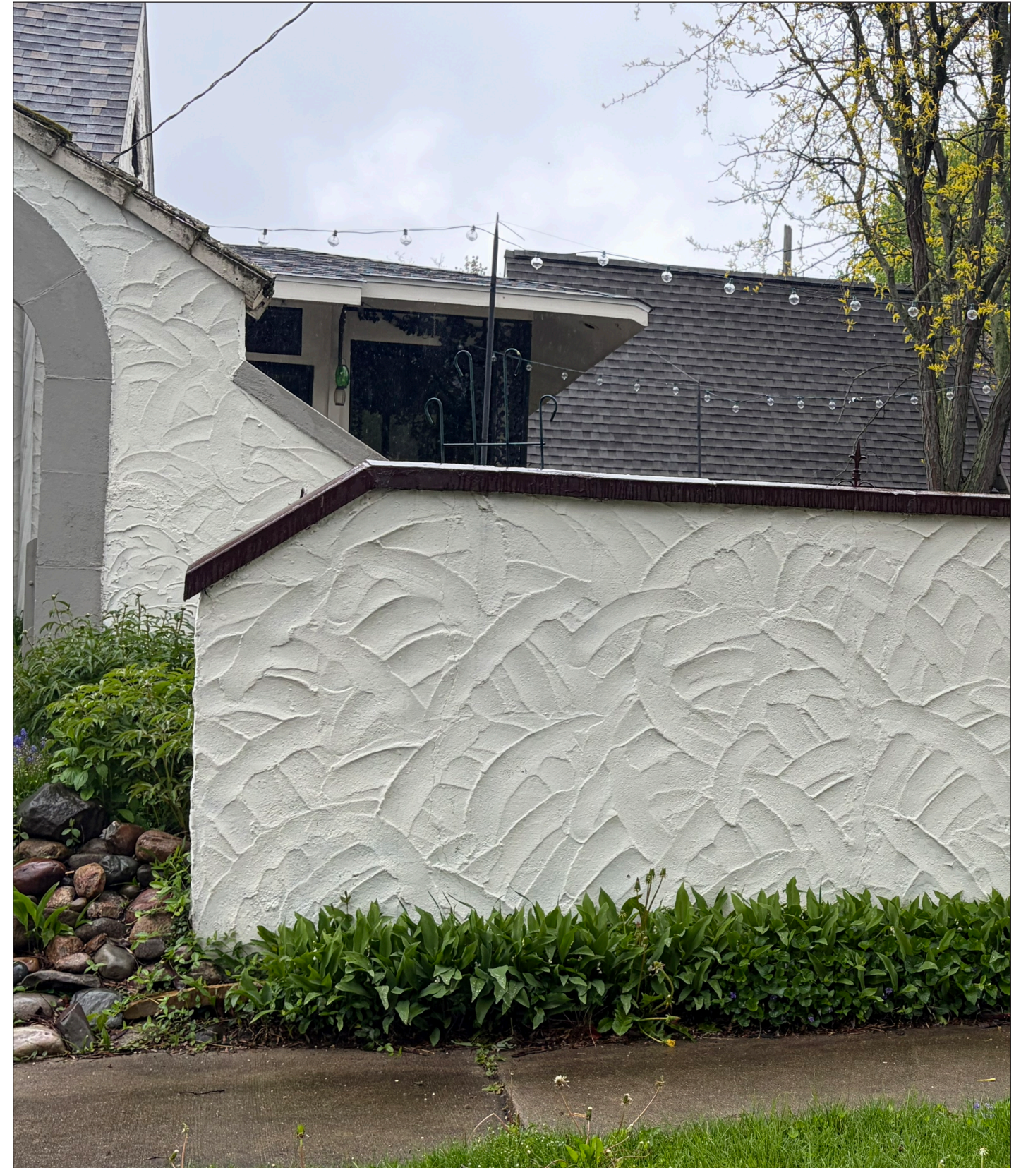
Stucco can be tooled into unique patterns as shown here. Masonry features like tooled stucco contribute to the historic character of the building and should be preserved. Photograph by Loggia Preservation, 2026.
