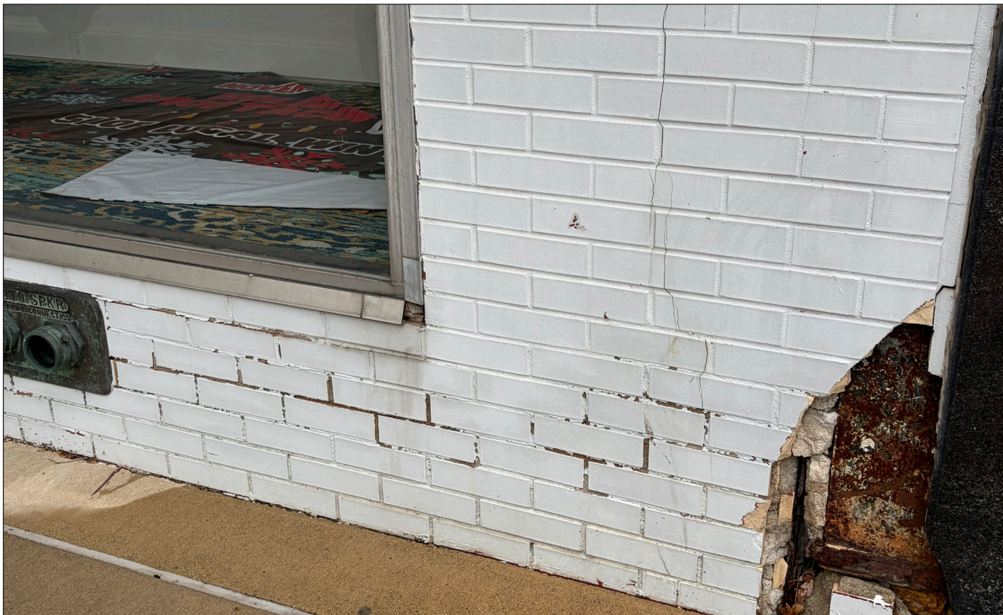
Unpainted brick is naturally porous which allows water and water vapor to pass through the brick; however, when brick is painted with latex paint, that process is compromised and water gets trapped in the brick which can cause significant damage to the masonry. Photograph by Loggia Preservation, 2026.
