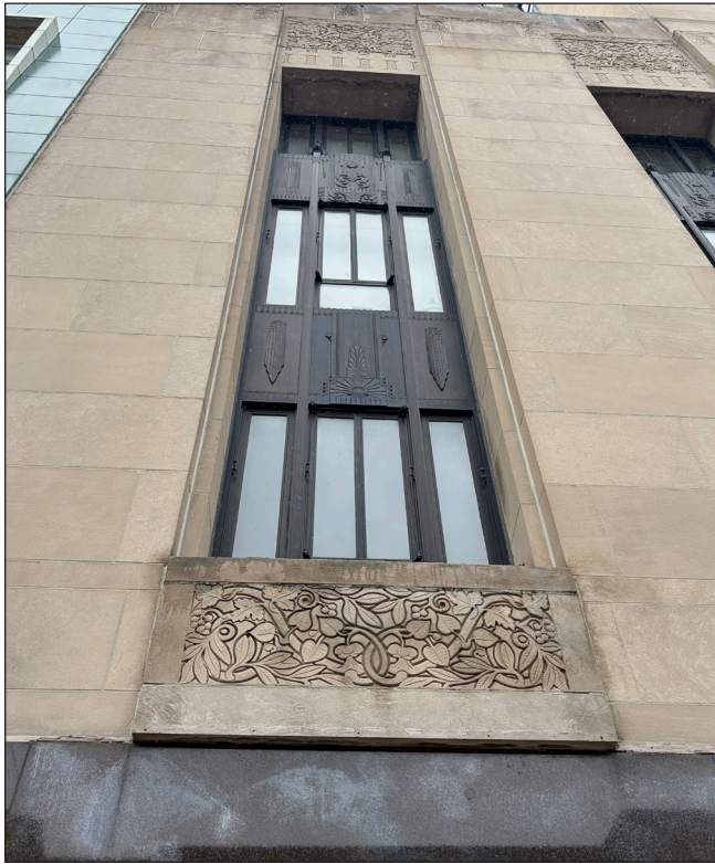
The carved limestone spandrel panels on the Milton Tower contribute historic character to the building and should be preserved. Photograph by Loggia Preservation, 2026.
