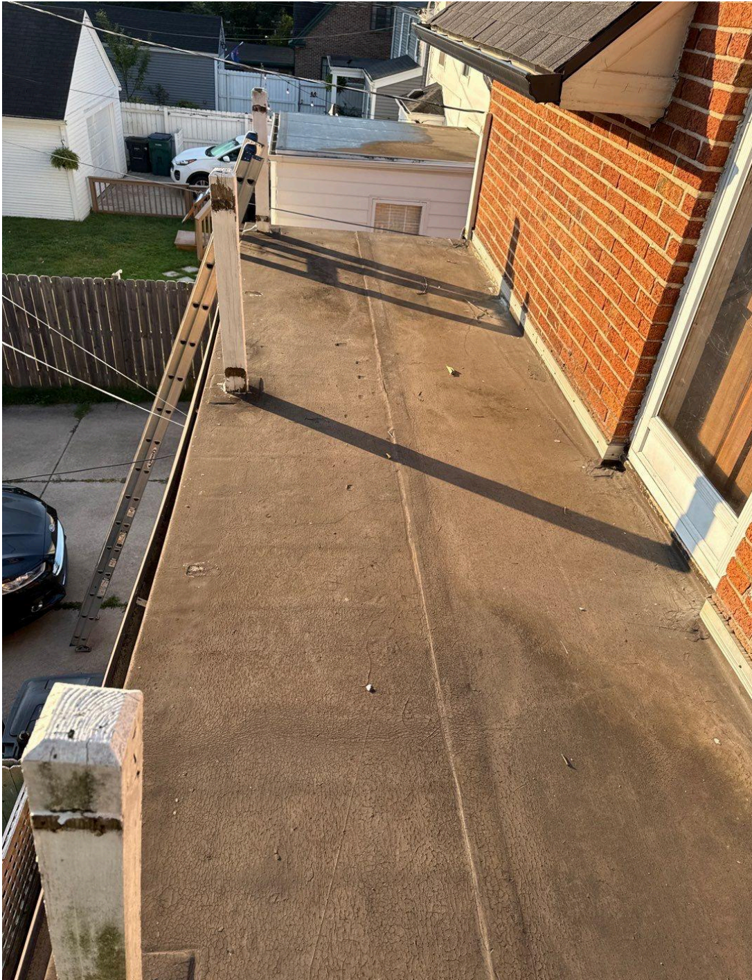
Flat roof that is being replaced – Homeowner already took down the railing
