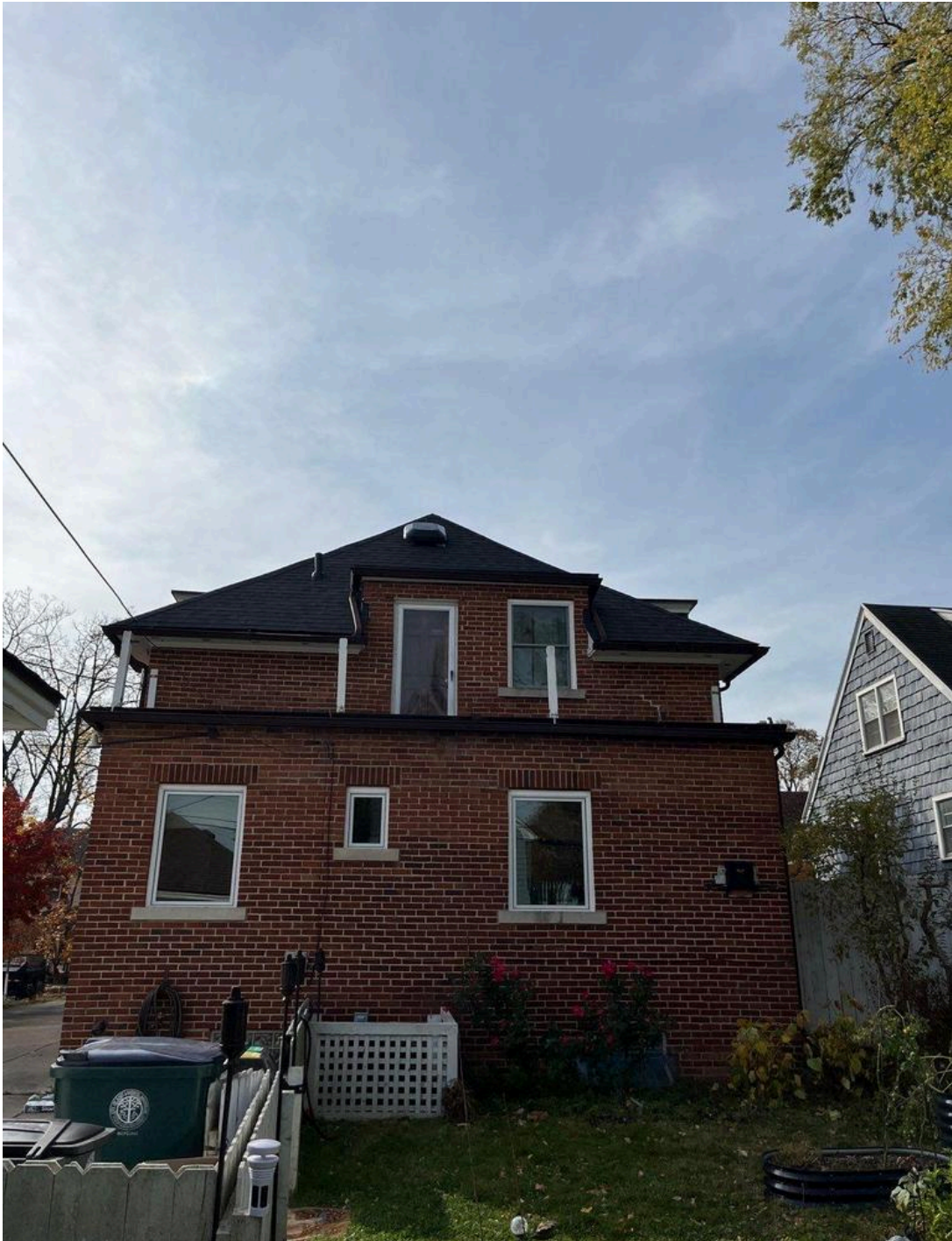
Flat roof that is being replaced – Homeowner already took down the railing - you can see posts
