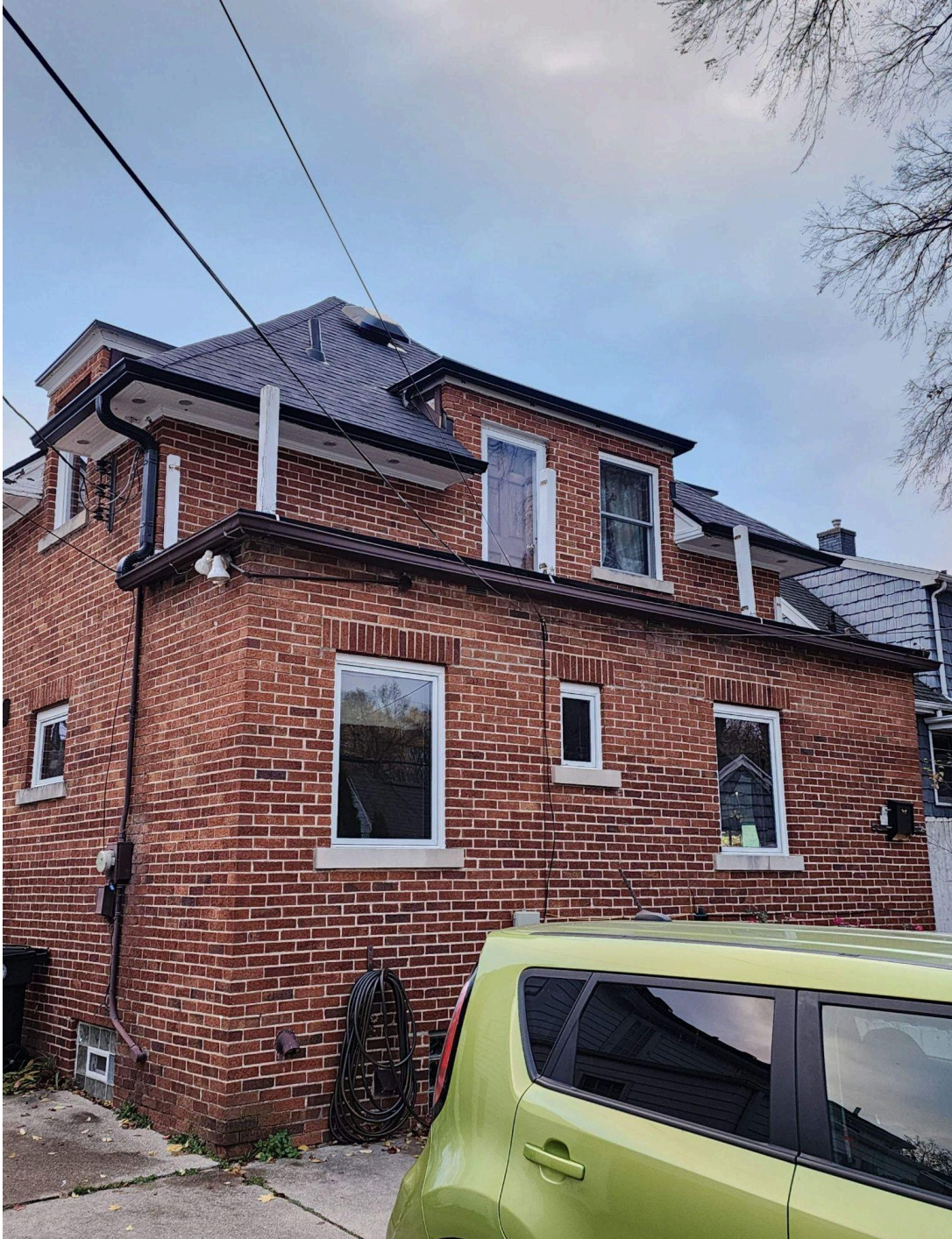
Flat roof that is being replaced – Homeowner already took down the railing - you can see posts
