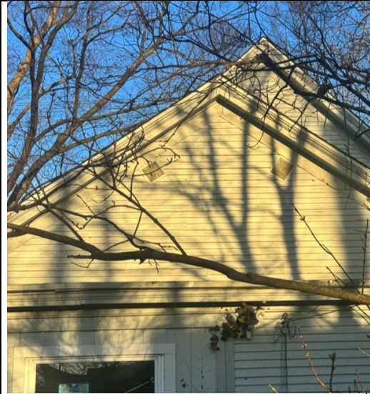
Figure 6: Close-up of the existing attic gable at the rear of the structure, showing the low, cramped profile of the current attic space.
