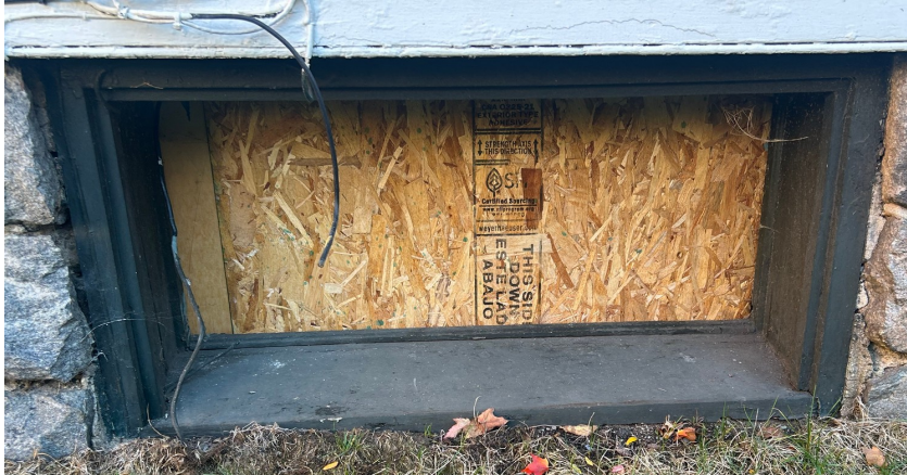
Degraded enclosure prior to restoration
