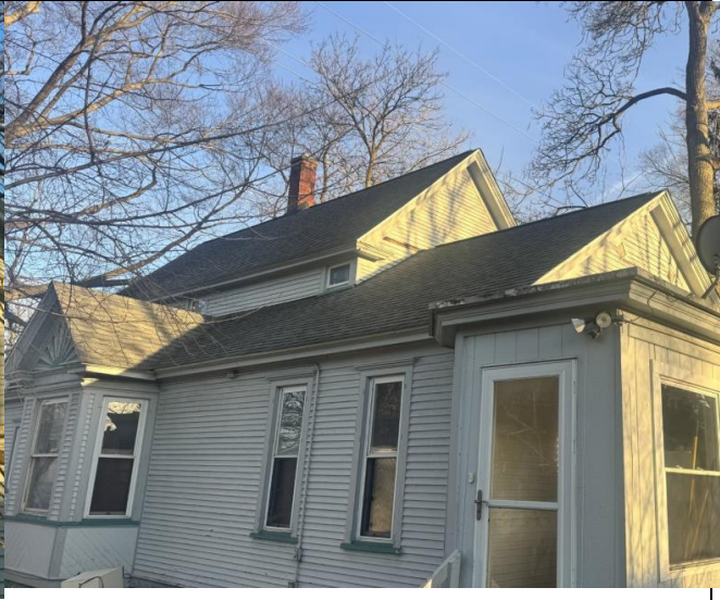
Figure 7: Full rear view showing the second-story attic roof (center) sitting visibly lower than the main house roofline, the area proposed for the addition.
