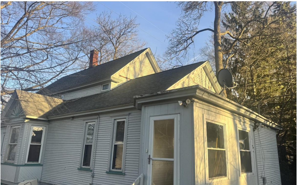
Figure 7: Full rear view of 276 Pine Ave, the lower attic roofline (center) sits significantly below the main roof peak. This is the existing structure that must be rebuilt and the area where the proposed addition will be located. Taken in winter when vegetation is absent; during the growing season this area is fully screened by trees.
