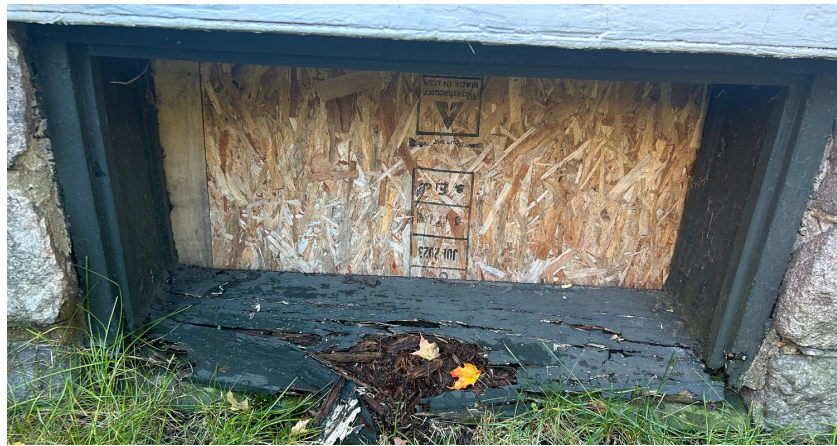
Degraded enclosure prior to restoration
