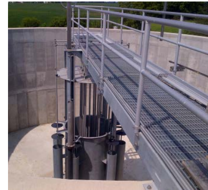
Post-Aerobic Digestion System
