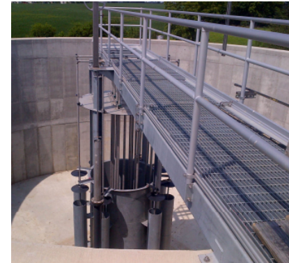
Post-Aerobic Digestion System
