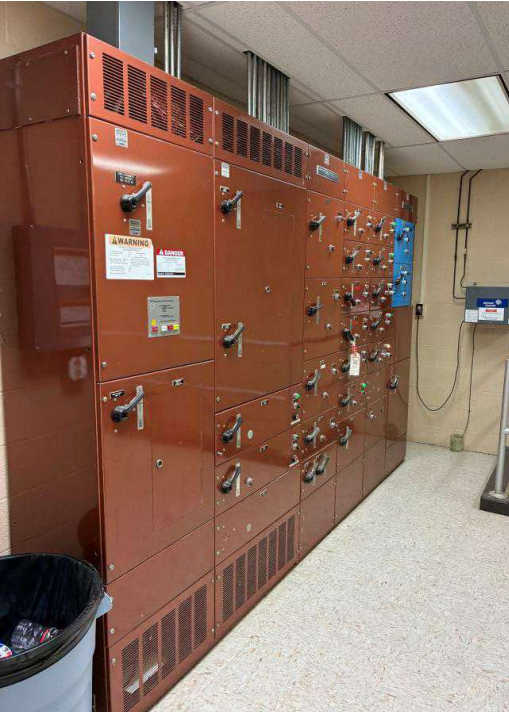
1970s era motor control center (MCC)
