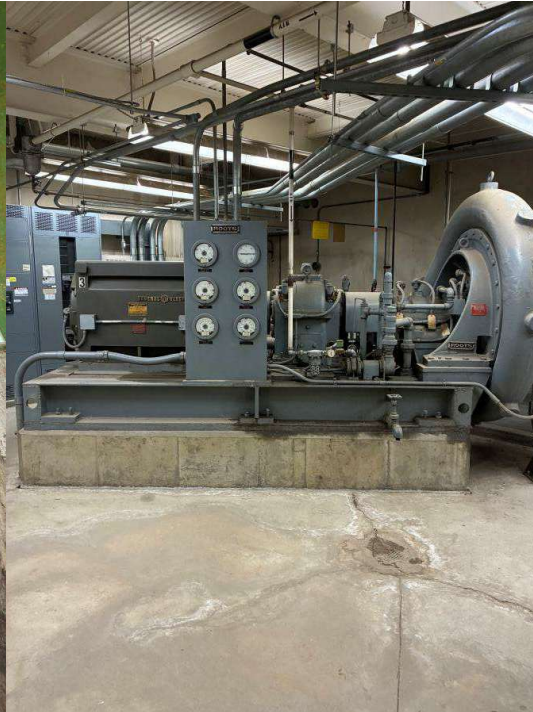
1970s era aeration blower
