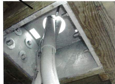
Fabricated metal box fastened between joists, flush with decking for mounting light poles on top.
