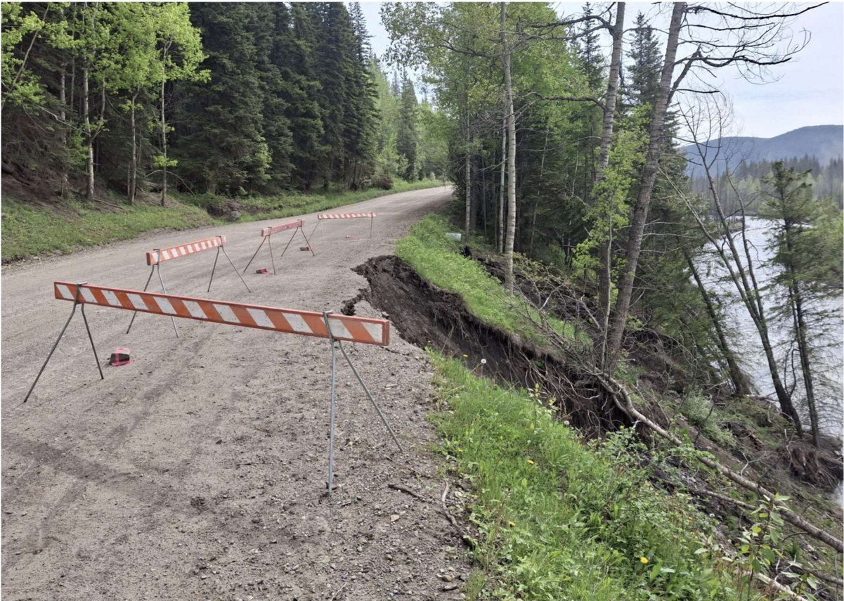
Northfork Road – km 65 Road Should Failure
