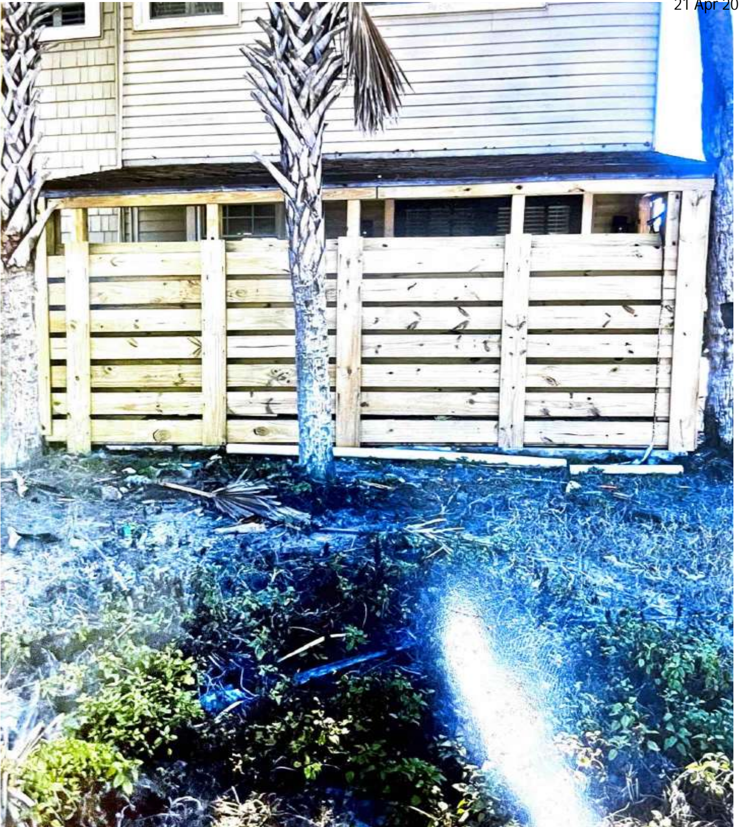
View of porch structure along rear property line
