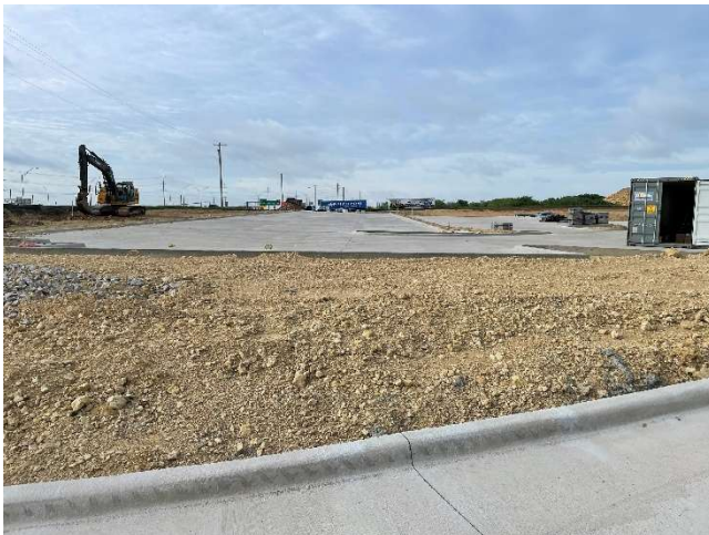
Site Improvements for Freeman Toyota located east of Harmon Road and West of IH35W
