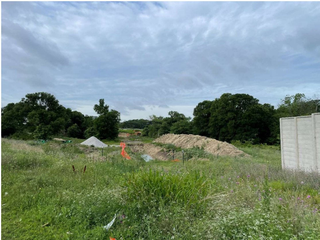
TRA/City Wastewater Interceptor Line Improvements adjacent to Stream HEN-2 under and north of Westport Parkway
