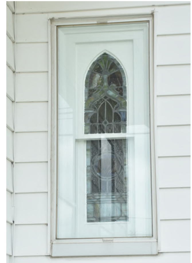
Existing stained glass windows are to remain, or to be salvaged and re-installed in new locations. New exterior storm panel are to be installed.
