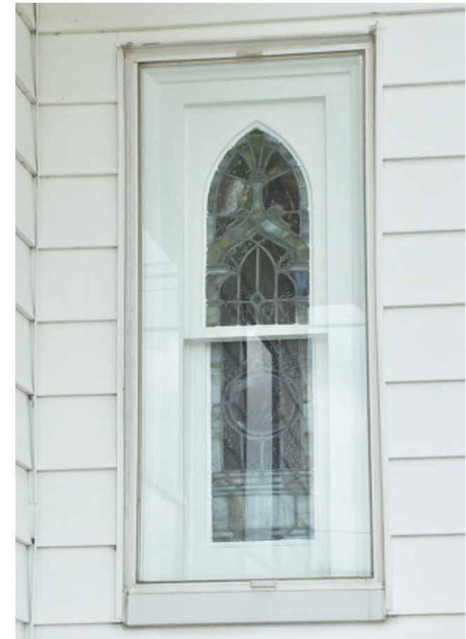
Existing stained glass windows are to remain, or to be salvaged and re-installed in new locations. New exterior storm panel are to be installed.
