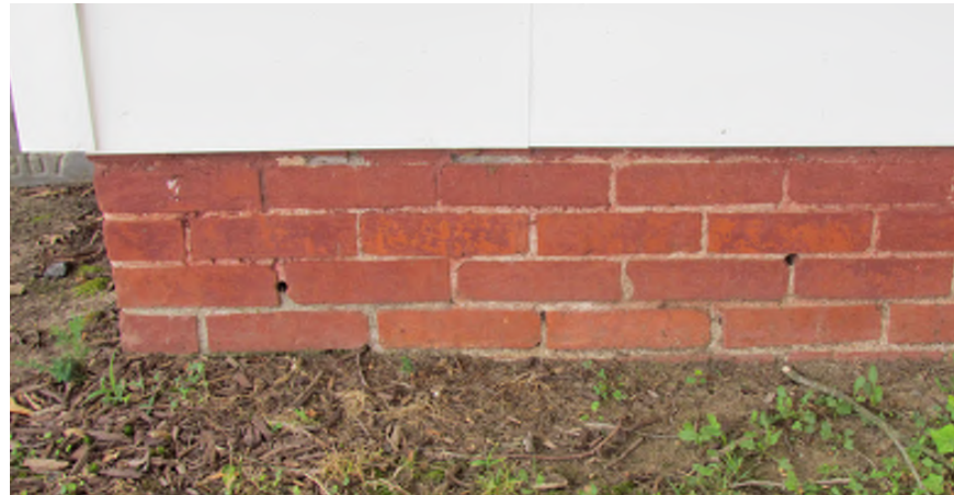
Brick and mortar at new foundations to match in size, color and pattern of existing brick.
