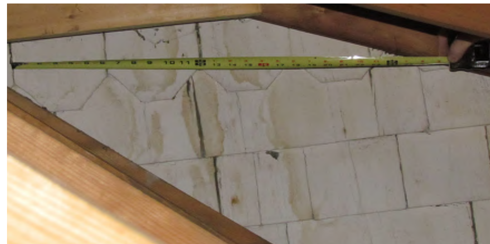
Original pattern shingles above square cut shingles as found within the attic space of 1960's addition.
