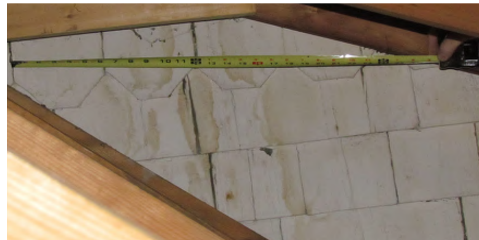
Original pattern shingles above square cut shingles as found within the attic space of 1960's addition.
