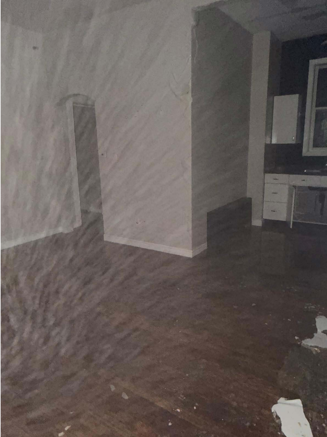
WATER DAMAGE 2026 – water & steam spraying from burst radiator
