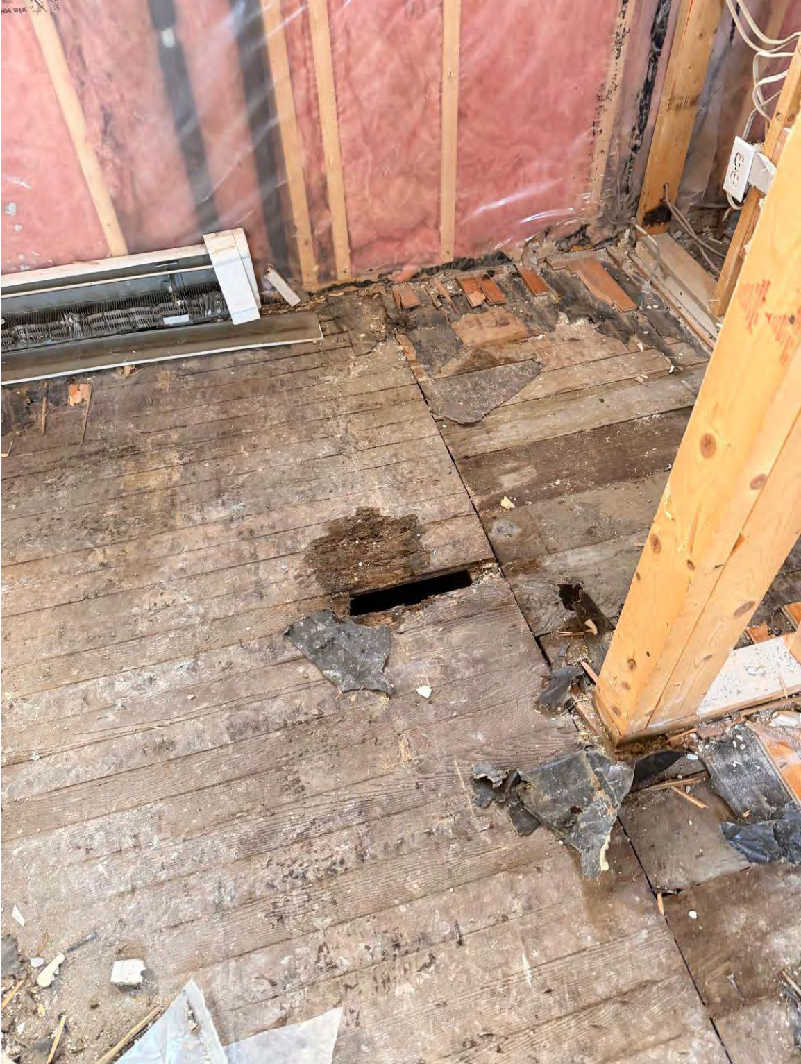
WATER DAMAGE 2026 – sections of subfloor in lower unit that fell into basement after standing water
