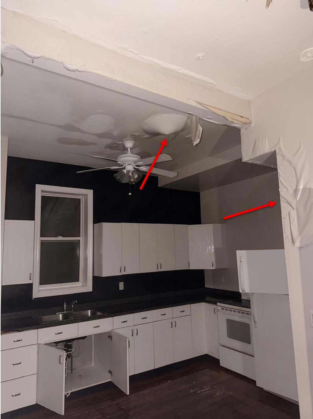
WATER DAMAGE 2026 - sagging paint due to water leak
