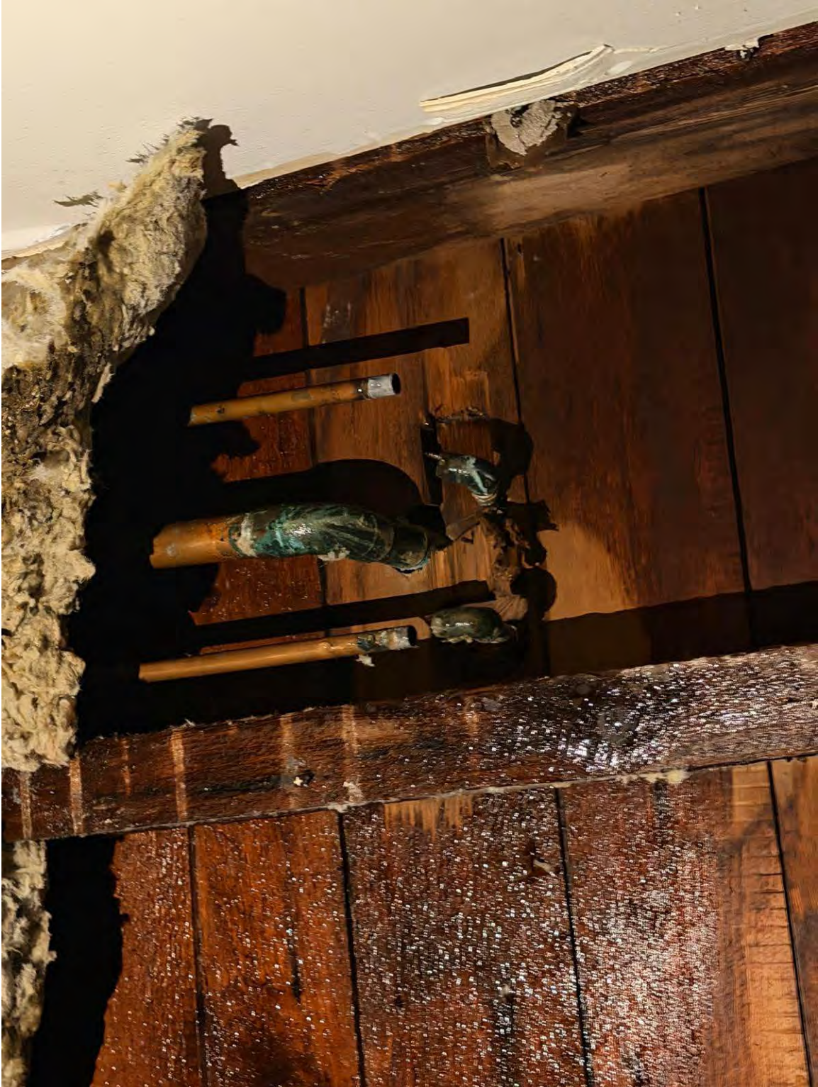
WATER DAMAGE 2026 – collapsed ceiling below burst pipe
