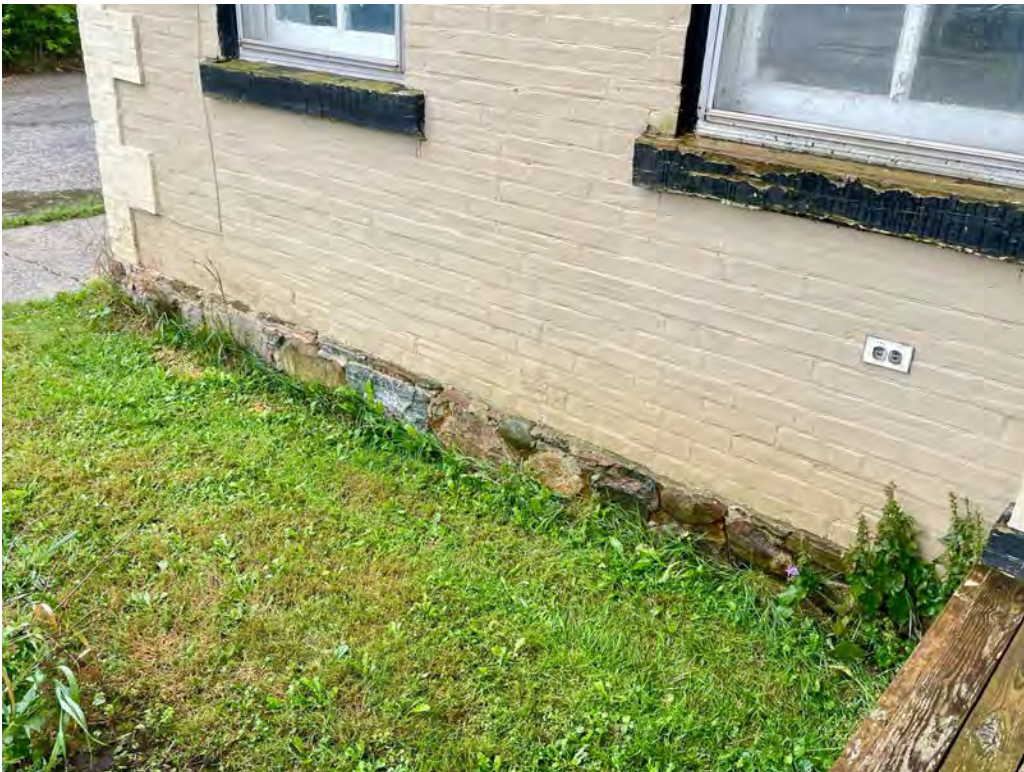
19 NELSON STREET WEST, FOUNDATION – there is a low foundation wall constructed of rubble
