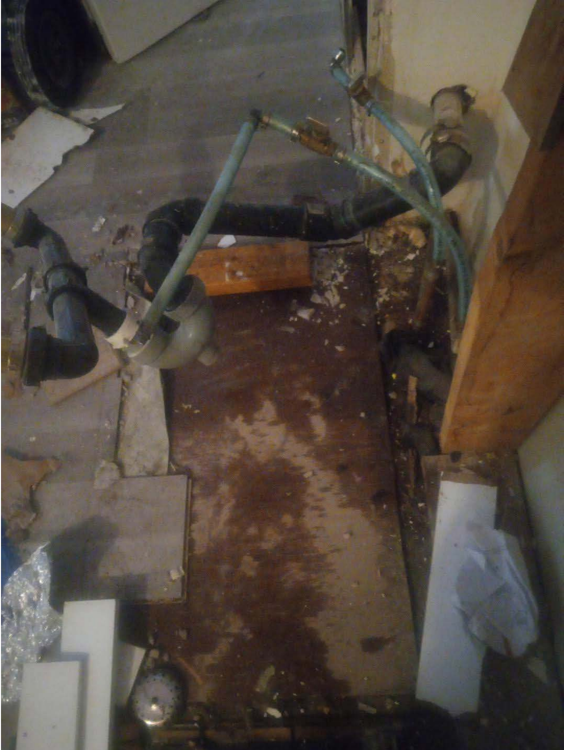
WATER DAMAGE 2026 – burst plumbing at downstairs washroom
