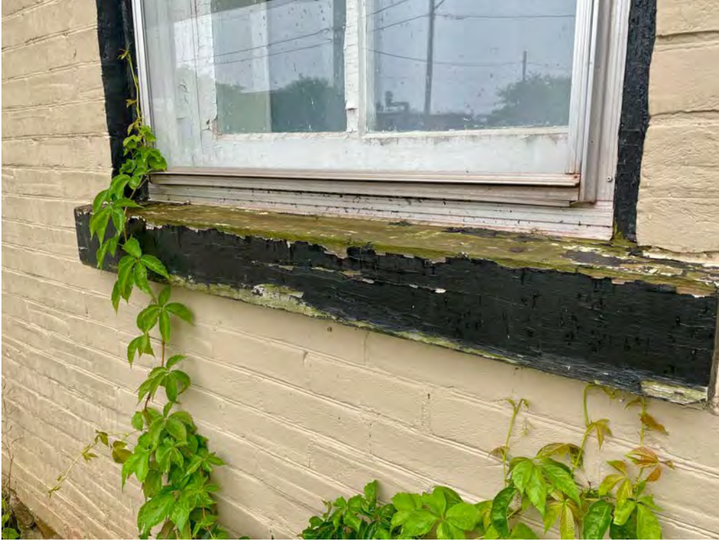
19 NELSON STREET WEST – the wood windowsills are in poor condition – the original 2 over 2 wood sash windows remain with modern aluminum storms installed on the exterior – the mortar joints have a beaded profile
