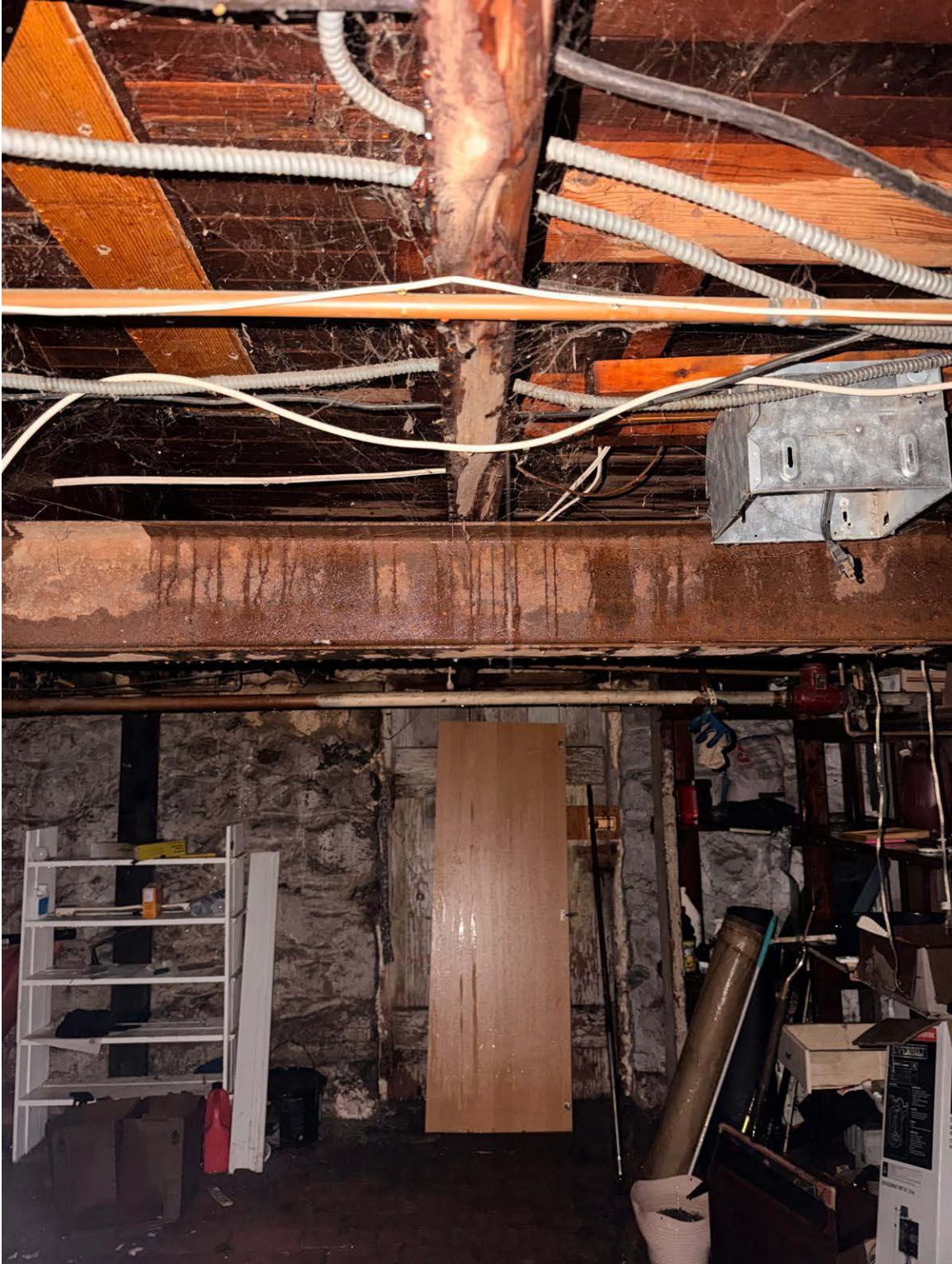
WATER DAMAGE – water pouring into basement below leak
