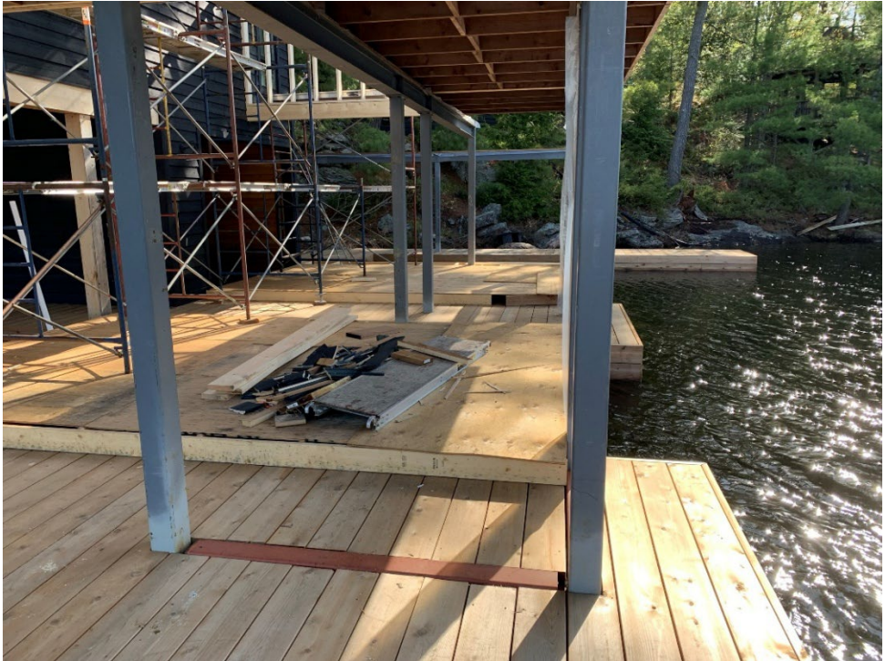
Figure 4: The southwest corner of the boathouse addition requiring relief.
