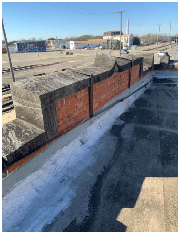
Roof: Modified Bitumen roof in good condition and in need of minor repairs. Flashing appears in fair condition
