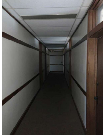
Second Floor: Sagging and stained ceiling tile indicating high humidity
