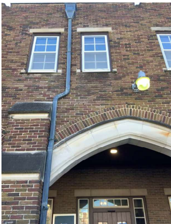
Exterior: Brick exterior is in good condition and in need of spot tuck pointing and sealant
