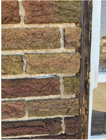
Exterior: Brick in need of tuck pointing and weatherproofing
