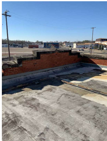
Roof: Modified Bitumen roof in good condition and in need of minor repairs
