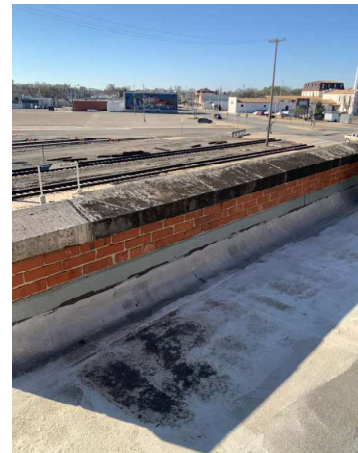
Roof: Brick wall and stone at parapet are in good condition, In need of sealant maintenance
