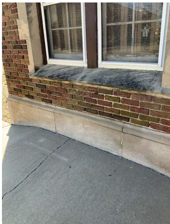
Exterior: Areas of tuck pointing and sealant
