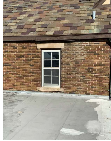
Exterior: Exterior brick in good condition and in need of spot tuckpointing. Some areas of wood rot need maintenance
