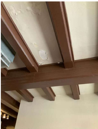
First Floor: Ceiling in need of paint and maintenance
