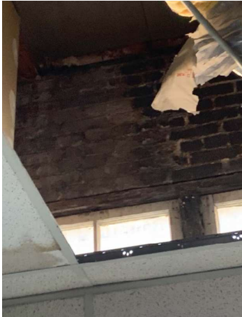
First Floor: Exterior wall repairs above lay-in ceiling system
