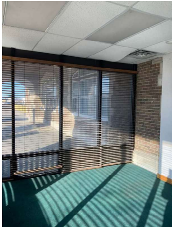
First Floor: Sagging ceiling tile indicating high humidity
