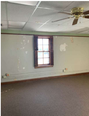
Second Floor: Exterior walls indicates moisture infiltration and in need of painting
