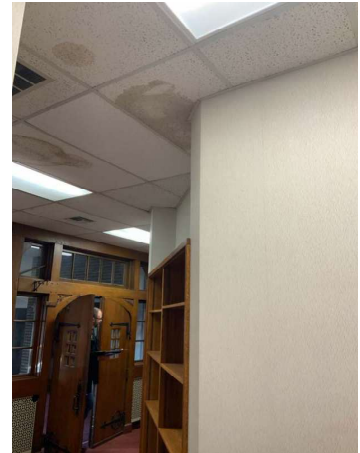
First Floor: Stained and sagging ceiling tile
