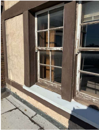
Exterior: Windows in need of sealant and caulking
