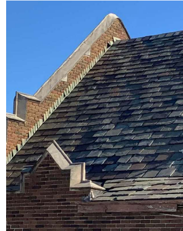
Roof: Slate tile roof in need of repair and replacement in areas
