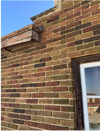
Exterior: Exterior brick in good condition and in need of spot tuckpointing. Some areas of wood rot need maintenance
