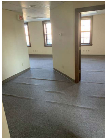
Second Floor: Carpet at end of life. Buckling indicates high humidity
