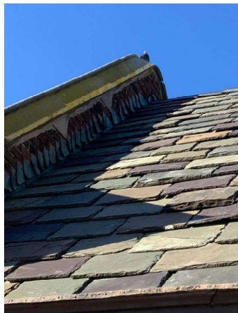
Roof: Slate tile roof in need of repair and replacement in areas. Flashing needs maintenance
