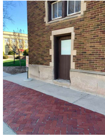
Exterior: Locations of deteriorated or damaged base stone
