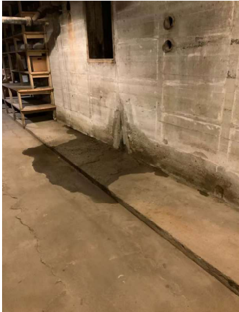
Basement: Ground water in basement area is limited. Sump pump appears operational
