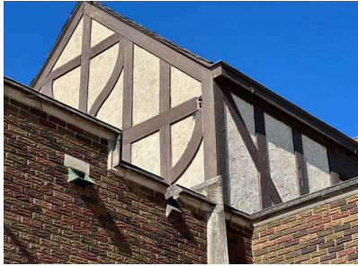
Exterior: Areas around building in need of wood trim repair and maintenance
