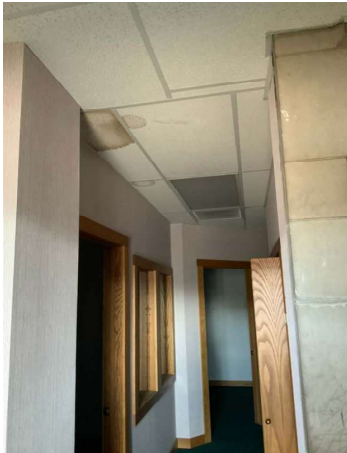
First Floor: Stained and sagging ceiling tile
