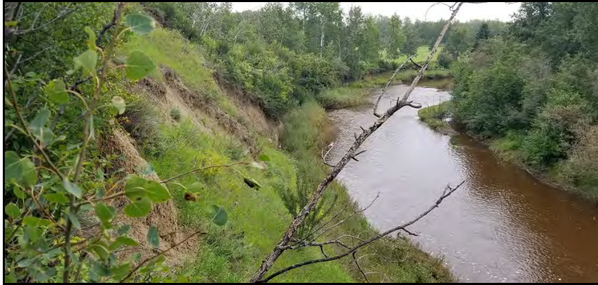
Photograph 4: Facing west from top of bank of steep hill at lower slopes, Heart River meander cutting into toe of slope.
