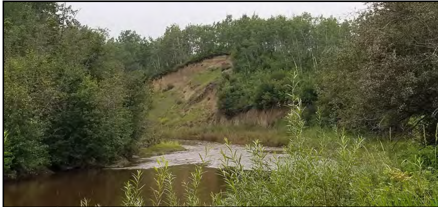
Photograph 5: Facing northwest towards steep hill at lower slopes, slope face stripped of vegetation indicating recent slope movement.
