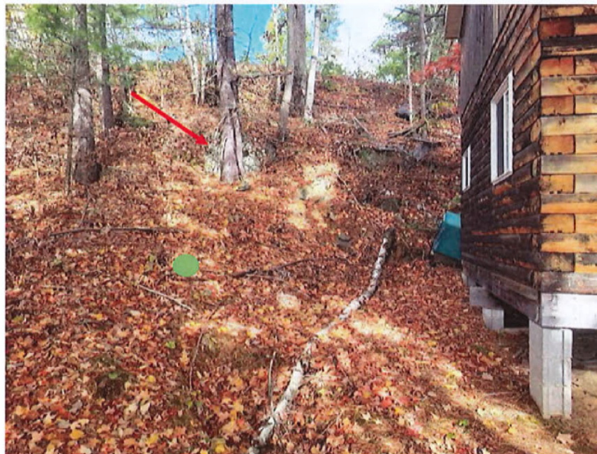
Photo 4 Middle of front slope – left side of cabin, October 2023.
