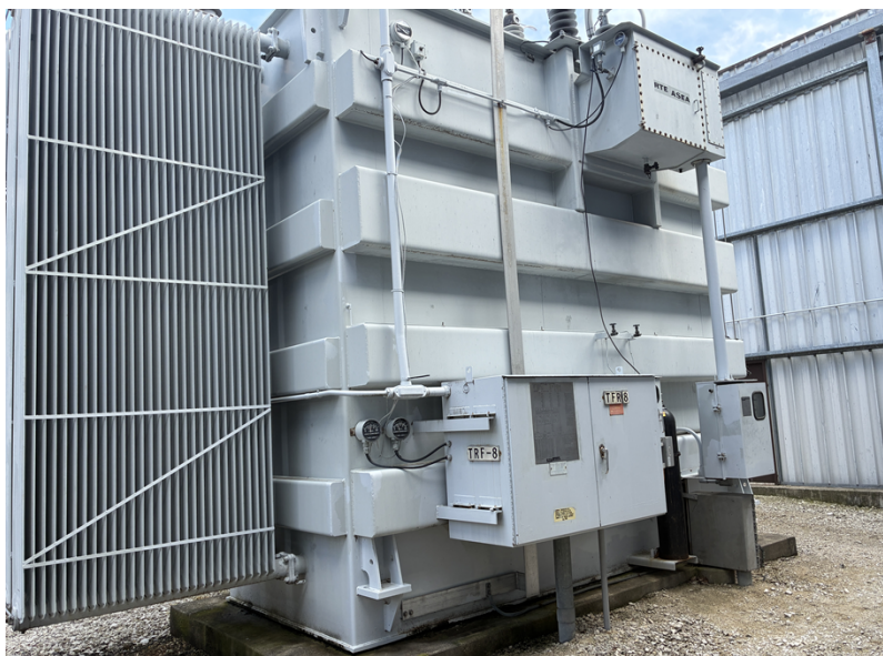
Existing Cooney SS Transformer – T8
