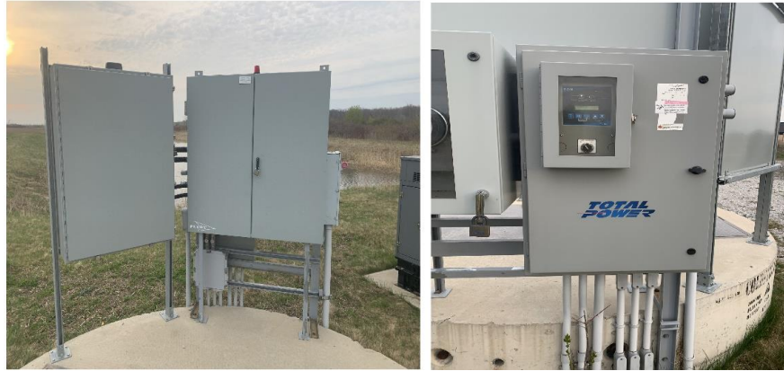
Figure 1 – Radcliff (Silver Springs) Pump Station Panels
