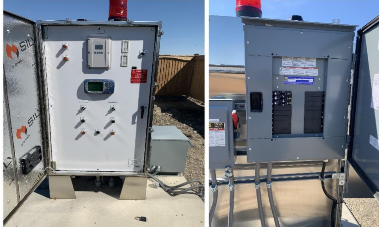
Figure 4 – Egremont Estates Pump Station Panel
