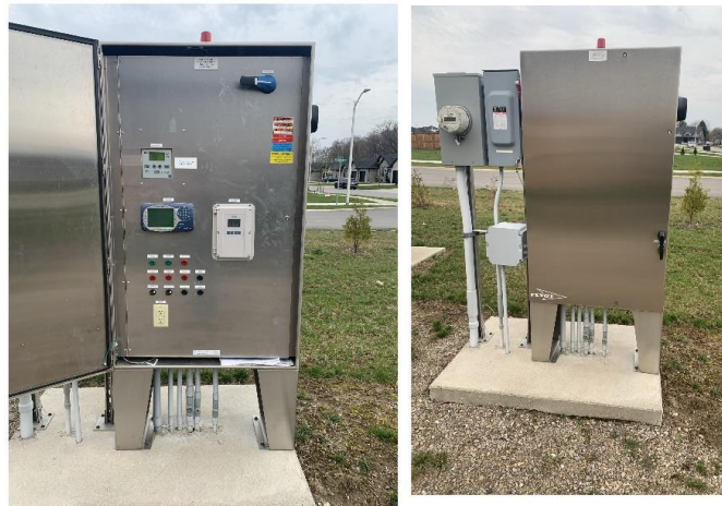
Figure 2 – Errol Woods Pump Station Panel
