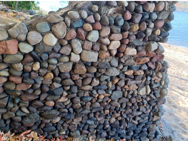
Figure 4 Fieldstone wall with worn mortar
