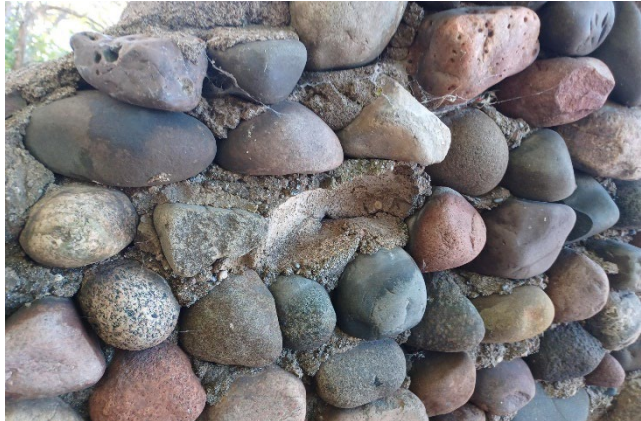
Figure 5 Stones falling out of fieldstone wall
