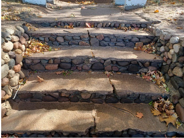
Figure 3 Cracking concrete stairs
