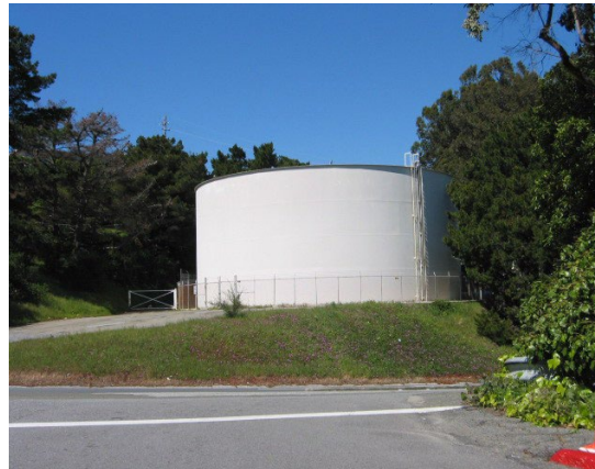
San Bruno's water supply comprises a blending of water from local wells and purchases from the San Francisco Public Utilities Commission. Municipal water is stored in eight storage tanks (shown) throughout the city.
