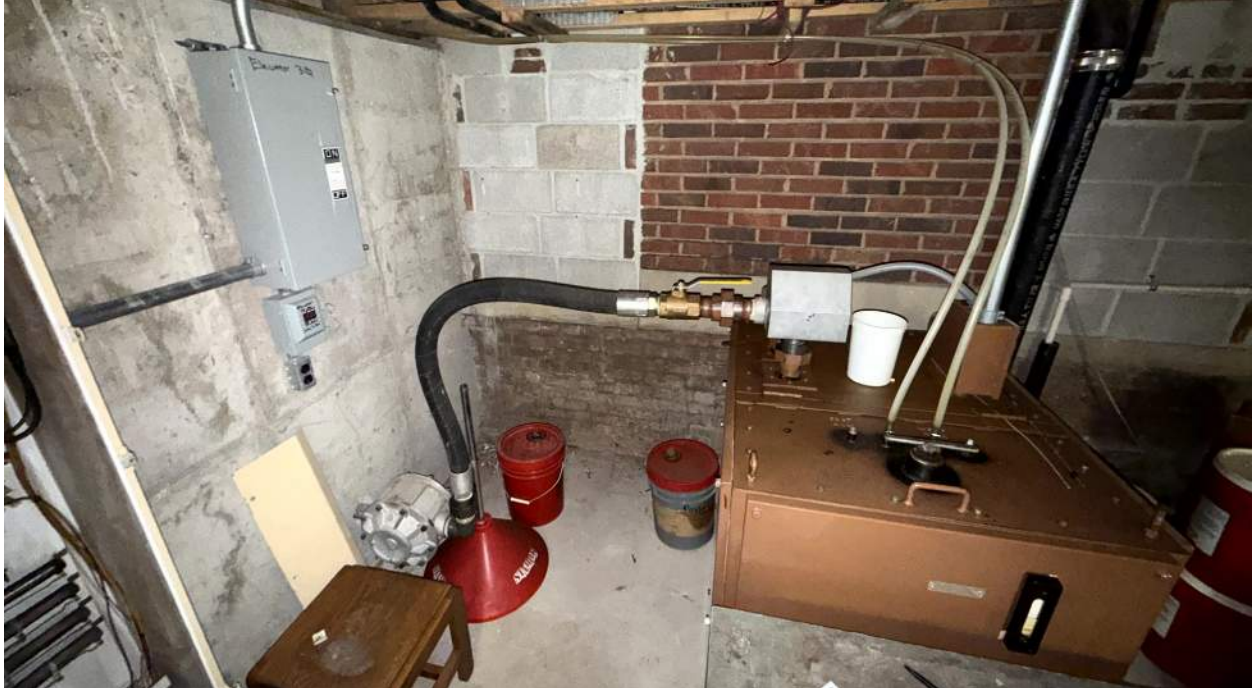
Elevator equipment and disconnect.
