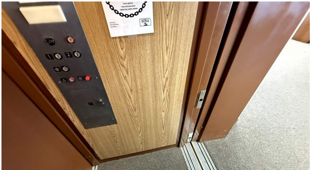
Elevator interior and controls.
