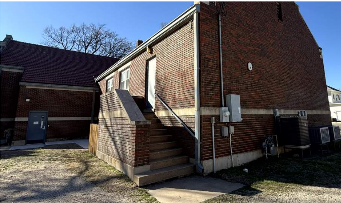
Accessibility barrier to upper floor (1982 additon)
