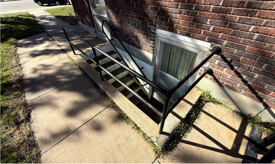
Accessibility barrier to lower floor (1917 construction)
