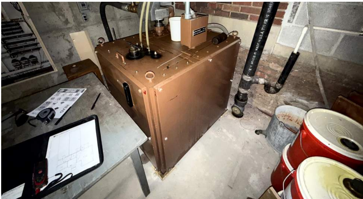
Elevator equipment and disconnect.
