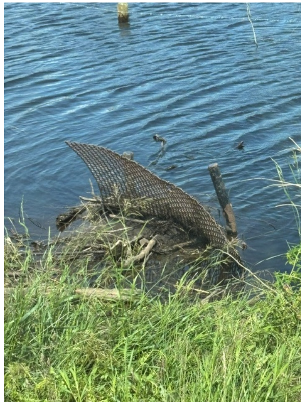
Public Works Figure 7.01. Dug Out Culvert/Beaver Dam
