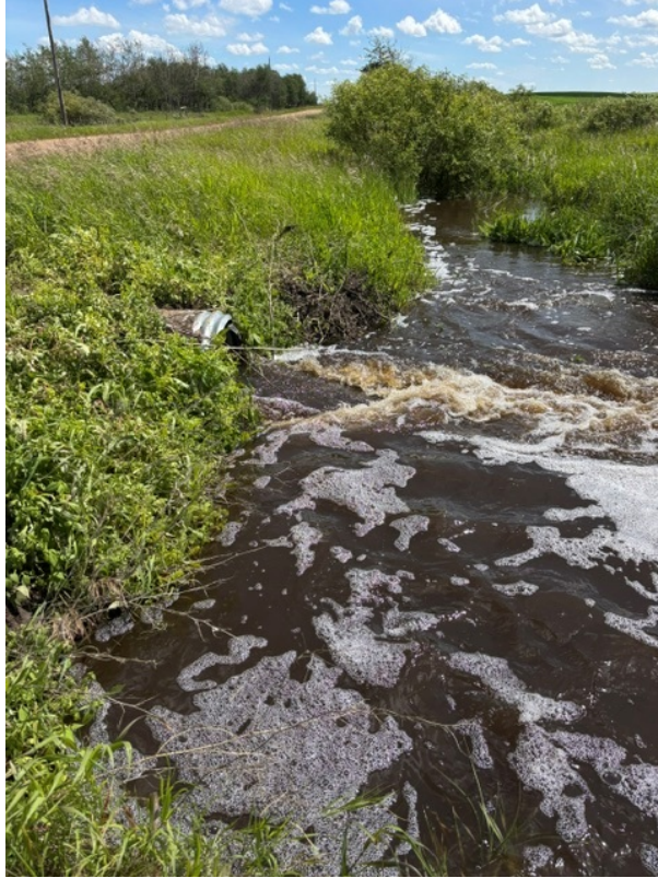
Public Works Figure 7.02. Dug Out Culvert/Beaver Dam
