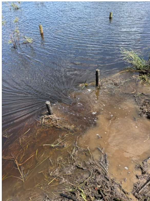
Public Works Figure 7.03. Dug Out Culvert/Beaver Dam
