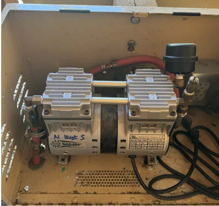
Projects, Engineering & Facilities Figure 1.01. Buffalo View Estates Aeration Motors Service & Re-Install
