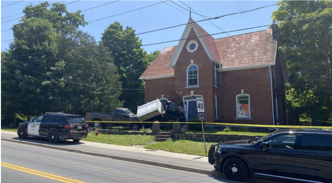
Figure 29 - Damage caused to a building in Sydenham, Ontario, due to a vehicle collision (Source: Vilela, 2023)
