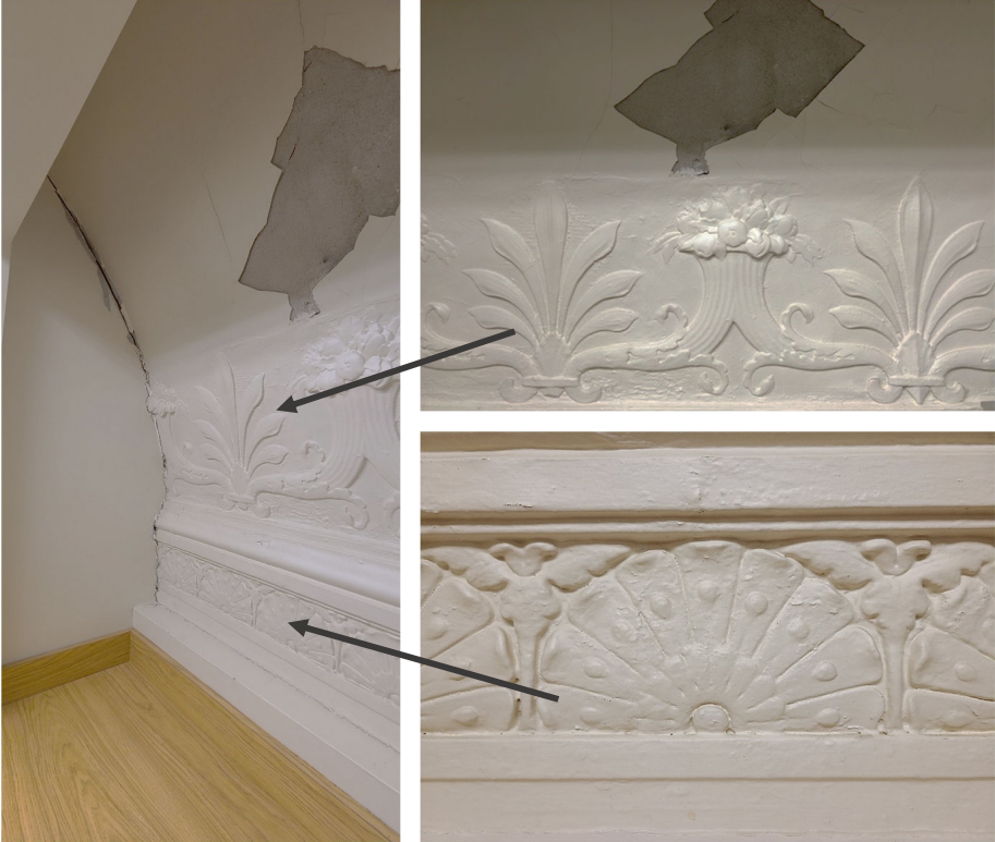
Photographs of plaster details on second floor which originally were part of wall decoration the the main hall. Photos: Nicola Alexander (2021)
