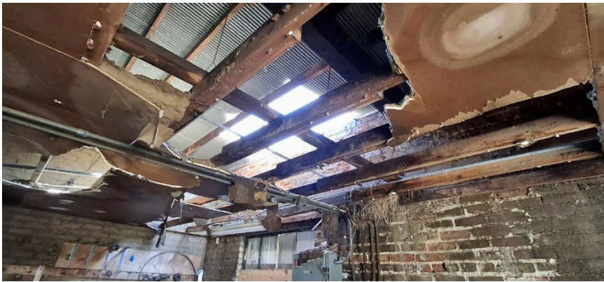
Railroad well house damage June 24 th 2026
