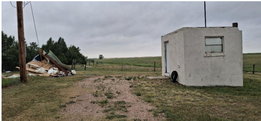
Atteberry well damage June 22 nd 2026
