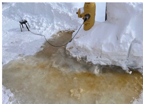
Hydrant 40 that began leaking during leak detection
