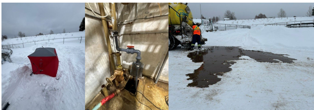
ClariPhos dosing tent
